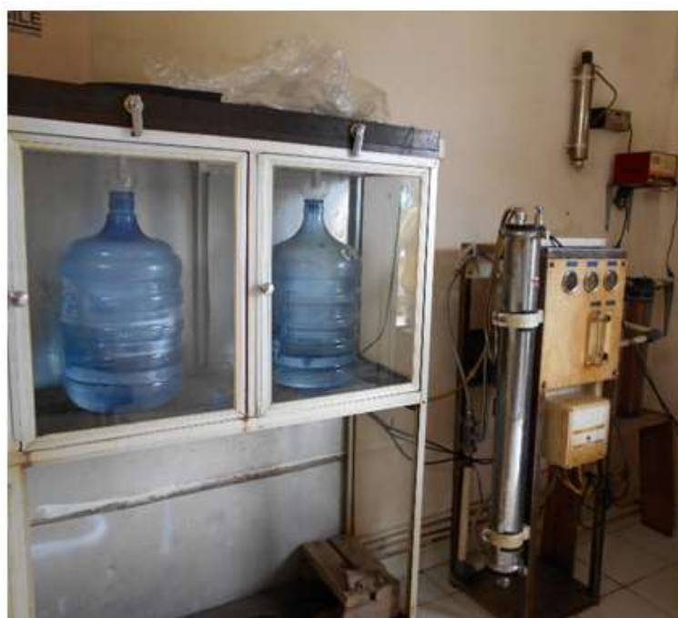
Gambar 4. Instalasi Pengolahan Air Minum Reverse Osmosis Sumber: PT. Nusantara Berau Coal, 2011 [22]
