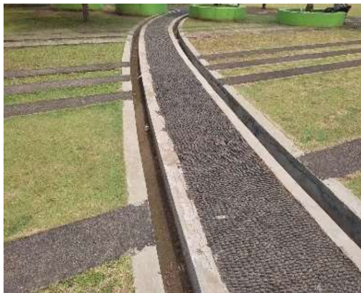
Figure 6. Uncovered drainage in Alun-Alun Kawali
