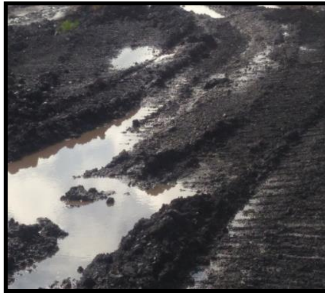
Gambar 3. Genangan Air Di area lantai Stockpile
